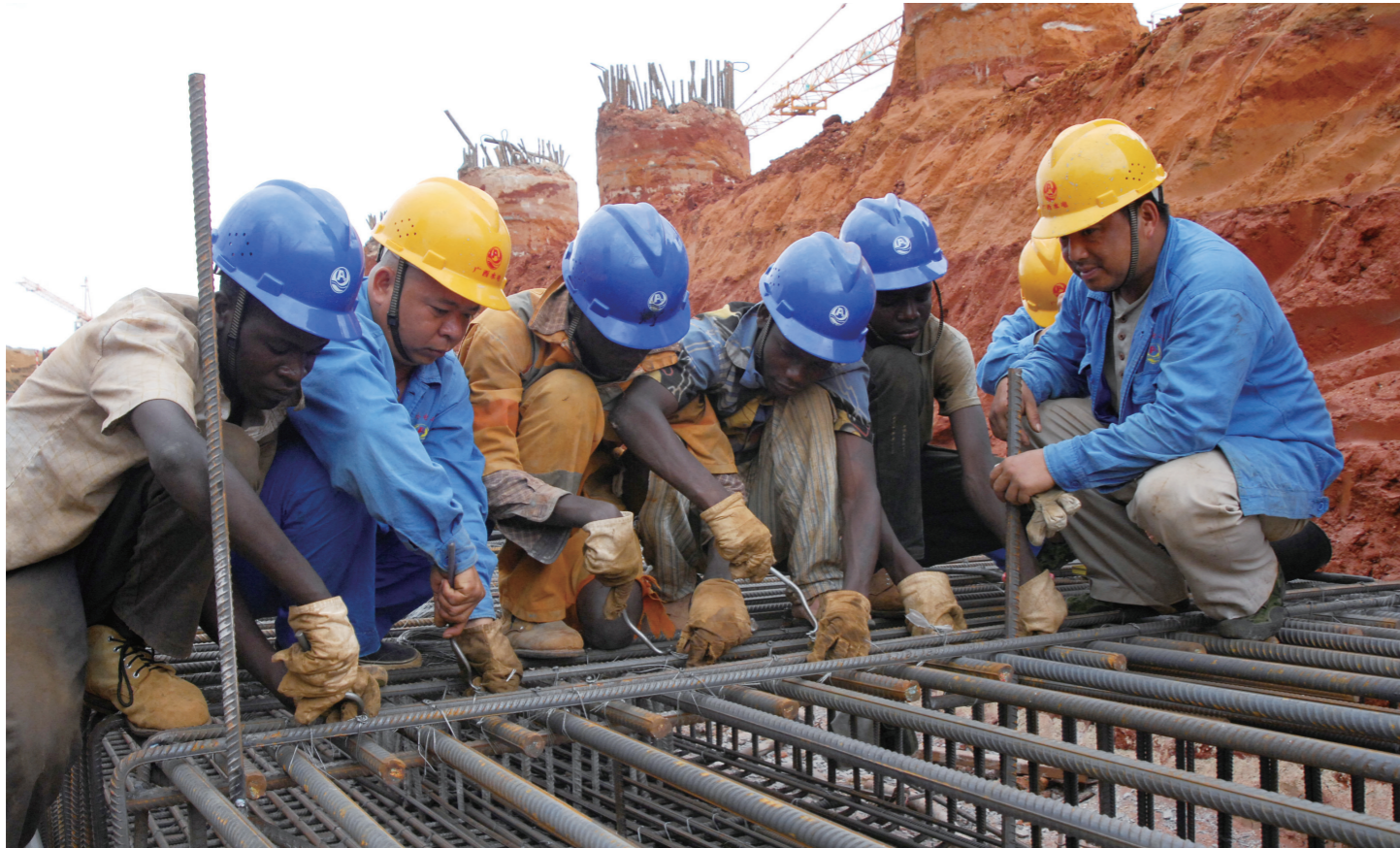
中方技术人员向当地员工教授钢筋绑扎技术 Chinese technicians taught local employees how to bind reinforced steel bars
